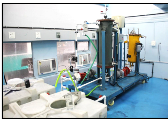
Fig. 5: Radiation grafted cellulosic adsorbent based semi pilot plant for dye waste water treatment
